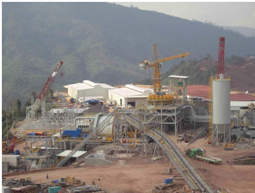
Phu Kham Copper-Gold Mine processing plant
