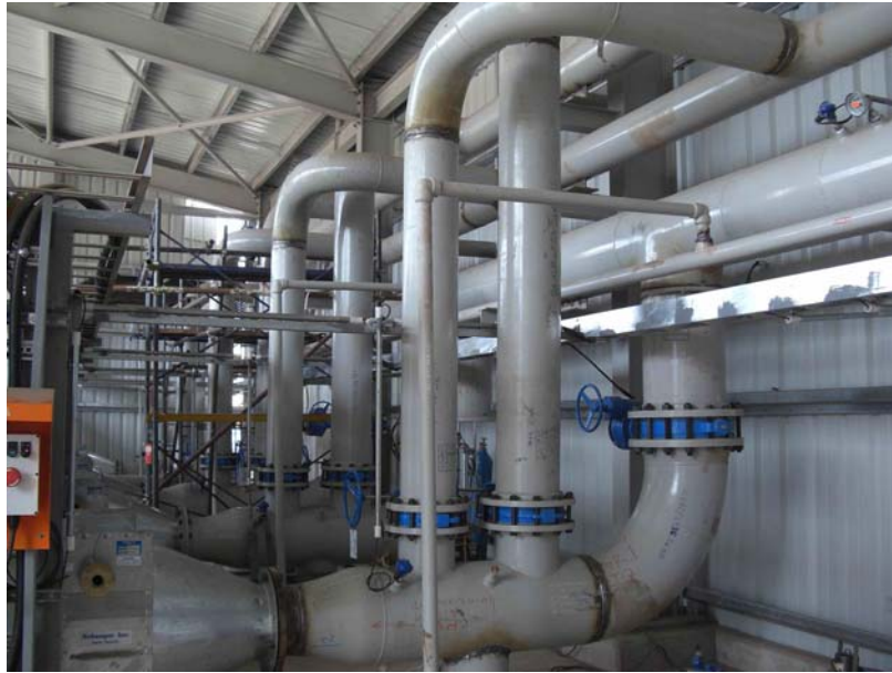
Flotation circuit blowers have been commissioned
